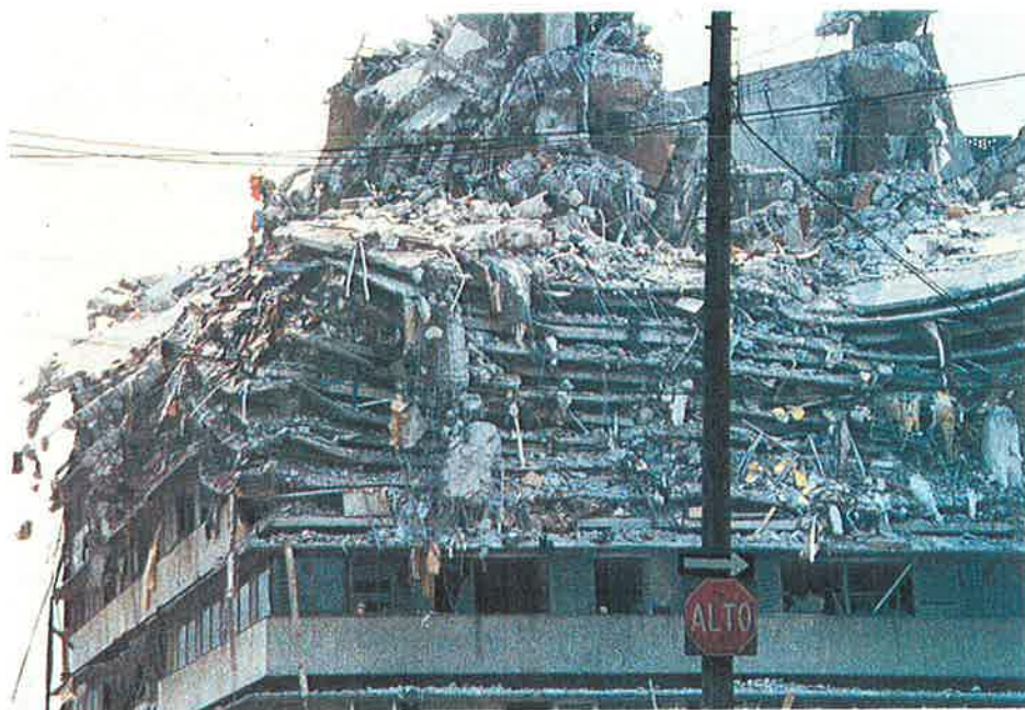
Remnants of Mexico City earthquake
